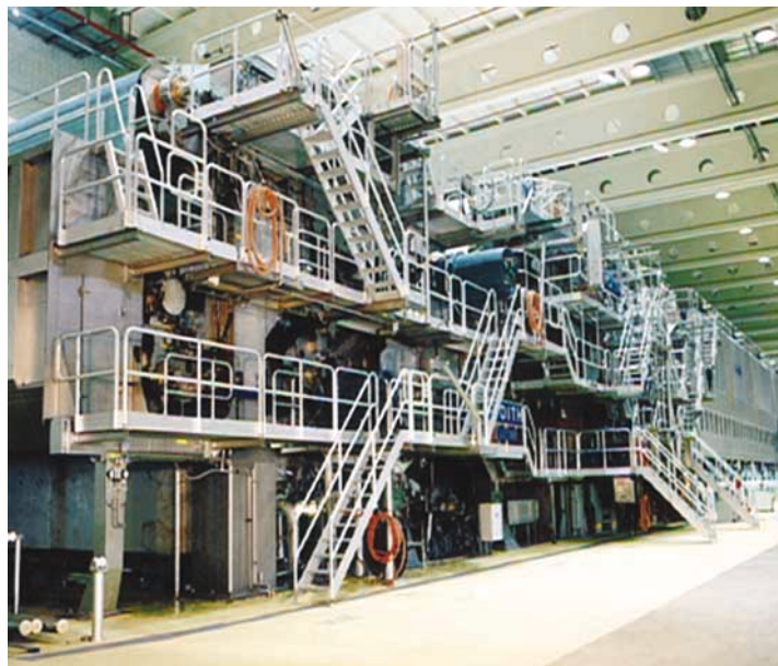
Figure 2: The paper production machine was commissioned in 1993
