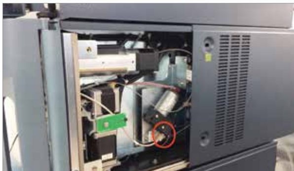
Figure 1. Side panel removal for sample manager wash tubing removal (fitting circled in red).
